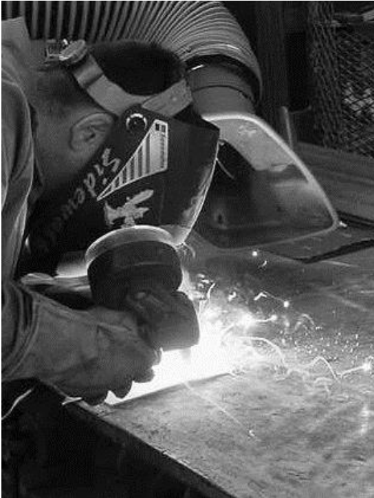
Welding Fumes Extraction
